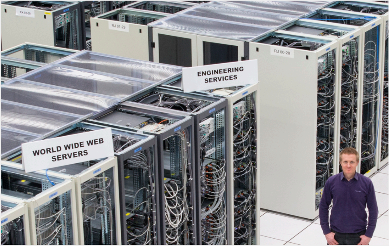
CERN data centre
